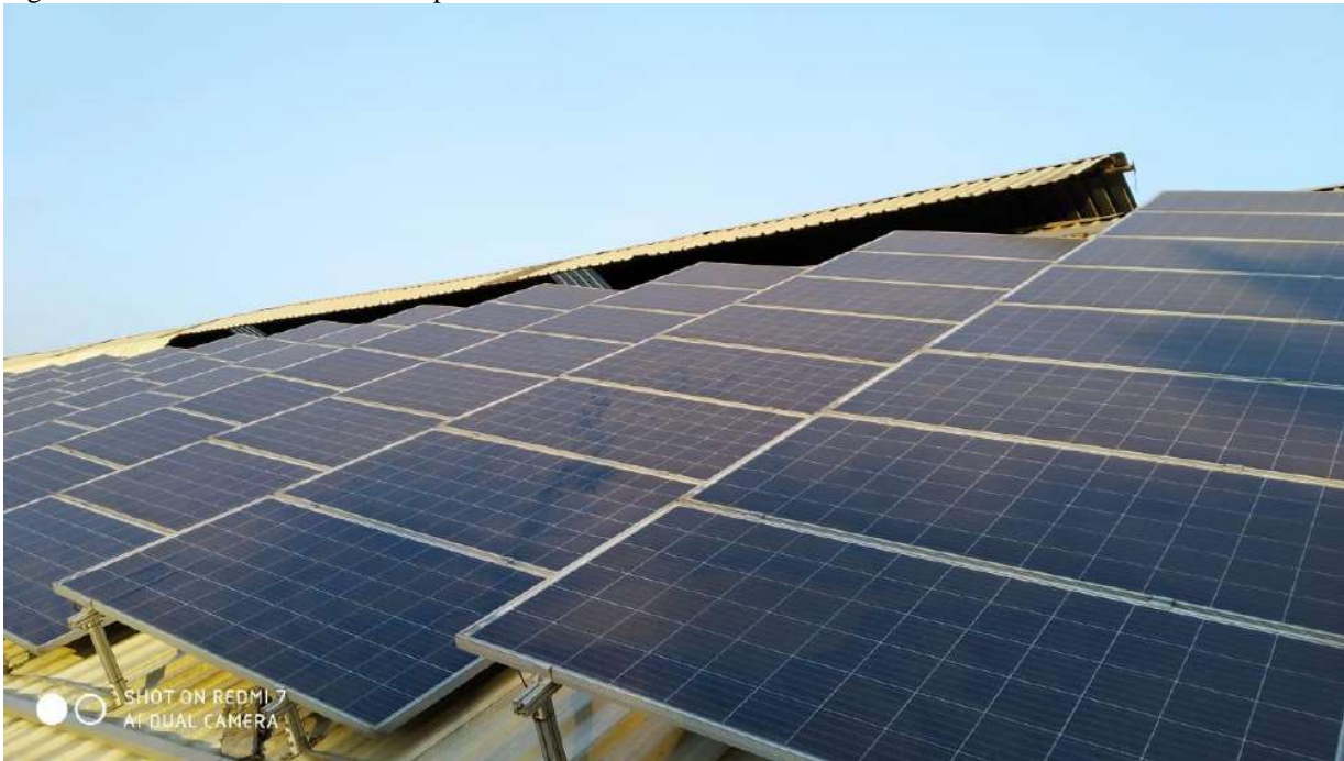
Fig-6: Solar Panels at CRC-1 roof top
