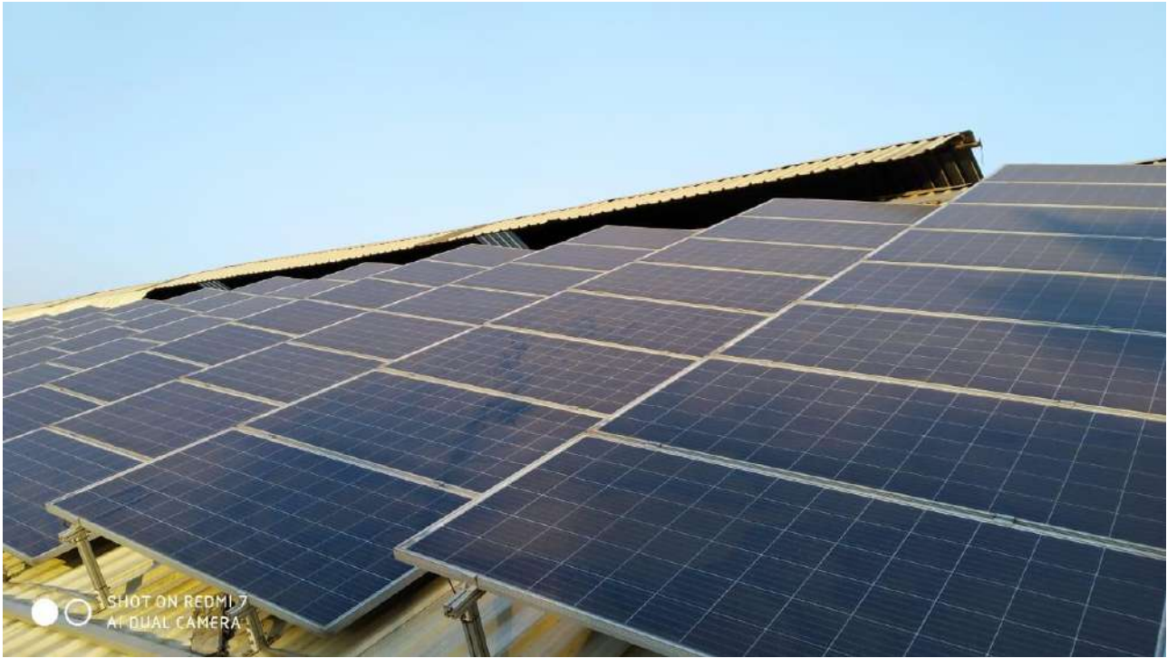
Fig-8: Solar Panels at MBA roof top:
