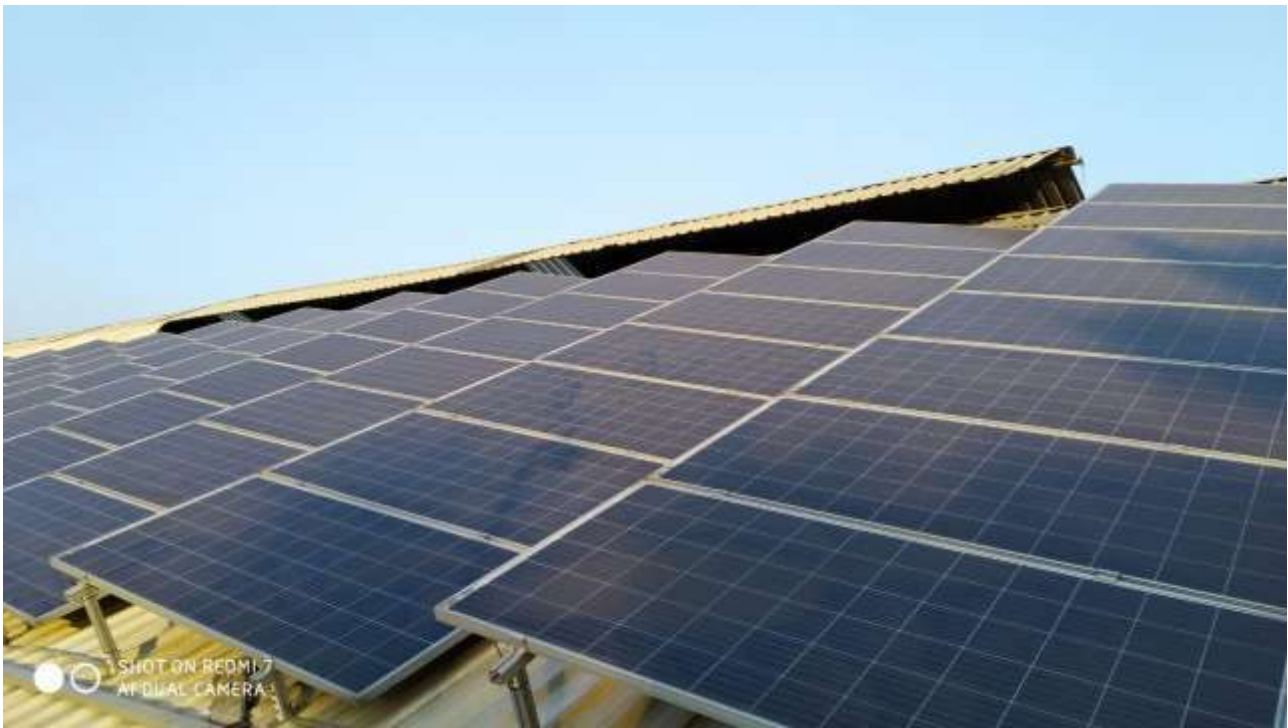
Fig-8: Solar Panels at MBA roof top:
