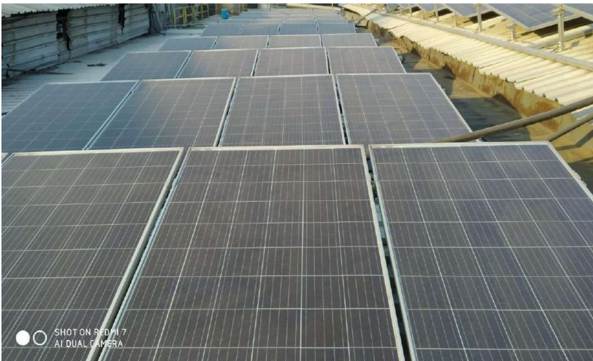
Fig-7: Solar Panels at CRC-2 roof top
