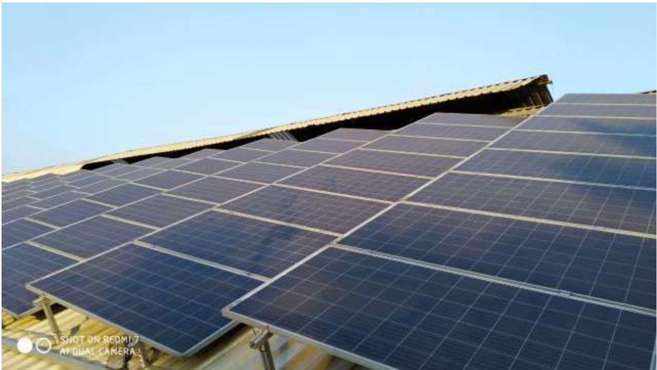
Fig-8: Solar Panels at MBA roof top:
