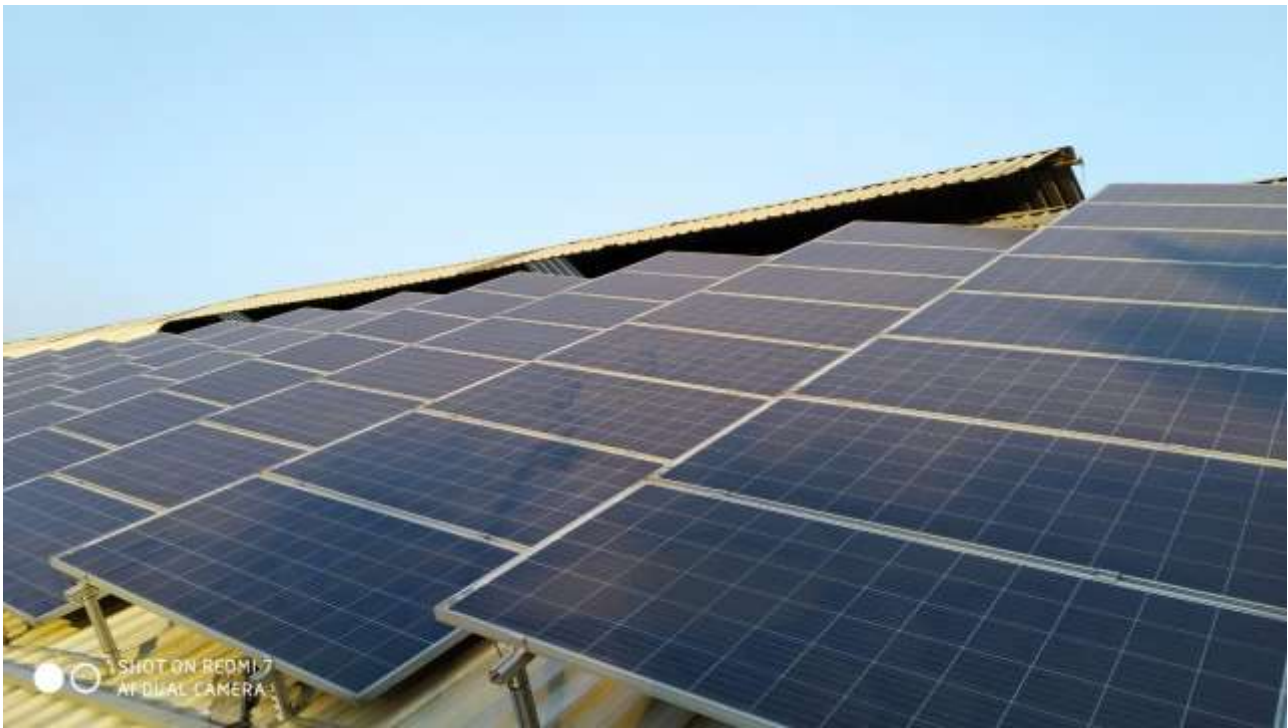
Fig-8: Solar Panels at MBA roof top:
