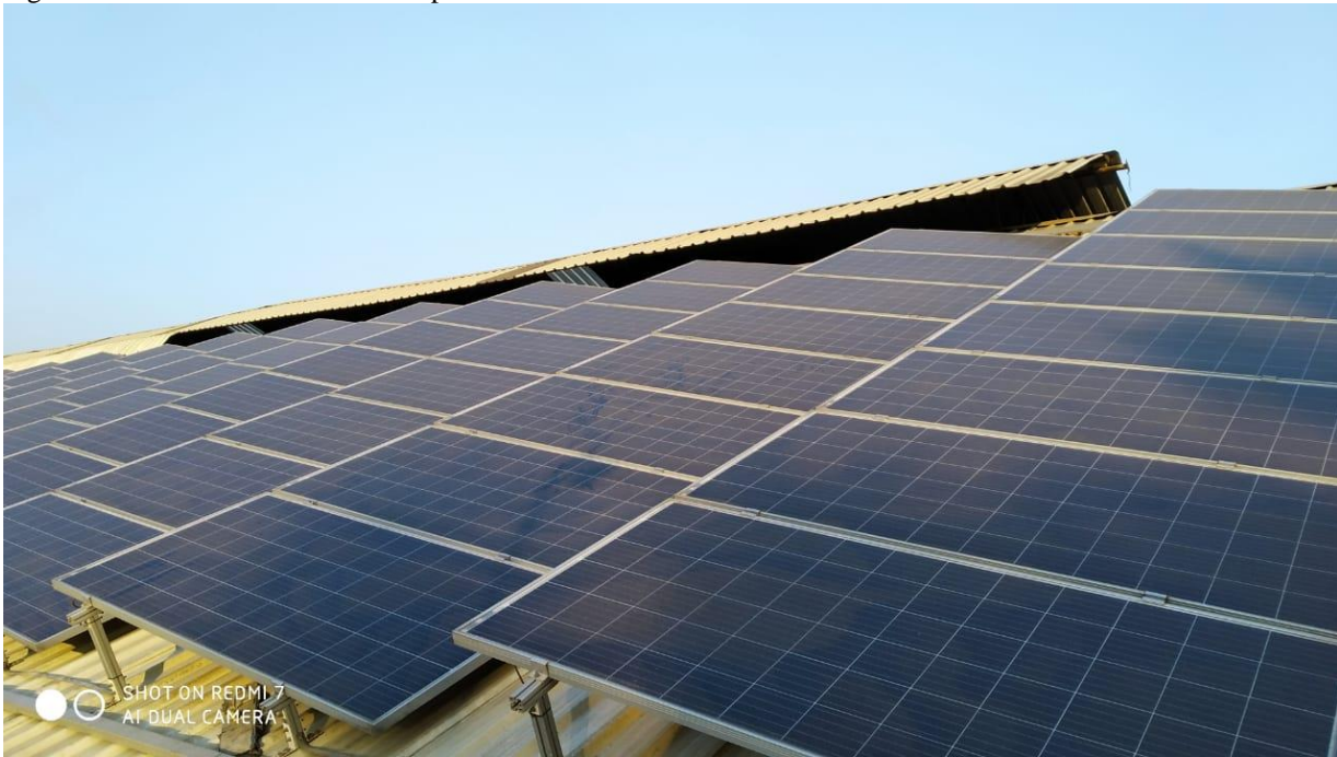
Fig-6: Solar Panels at CRC-1 roof top
