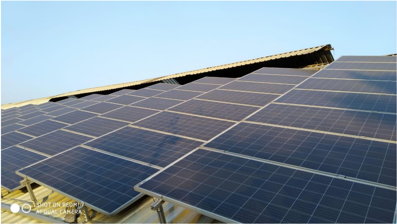
Fig-8: Solar Panels at MBA roof top:
