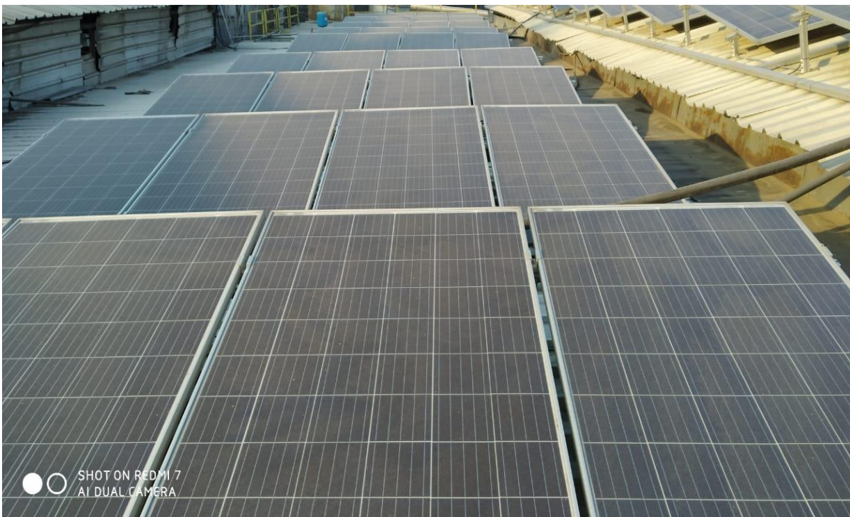
Fig-7: Solar Panels at CRC-2 roof top
