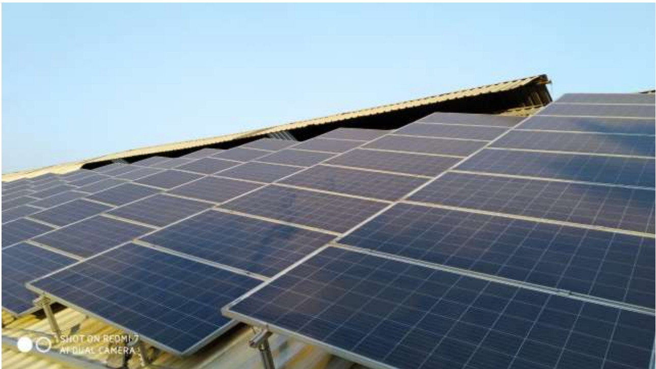
Fig-8: Solar Panels at MBA roof top:
