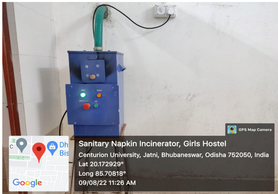
(Incinerator Bhubaneswar Campus)
