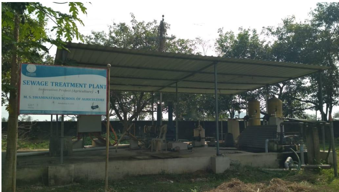
Figure 26: Sewage Treatment Plant
