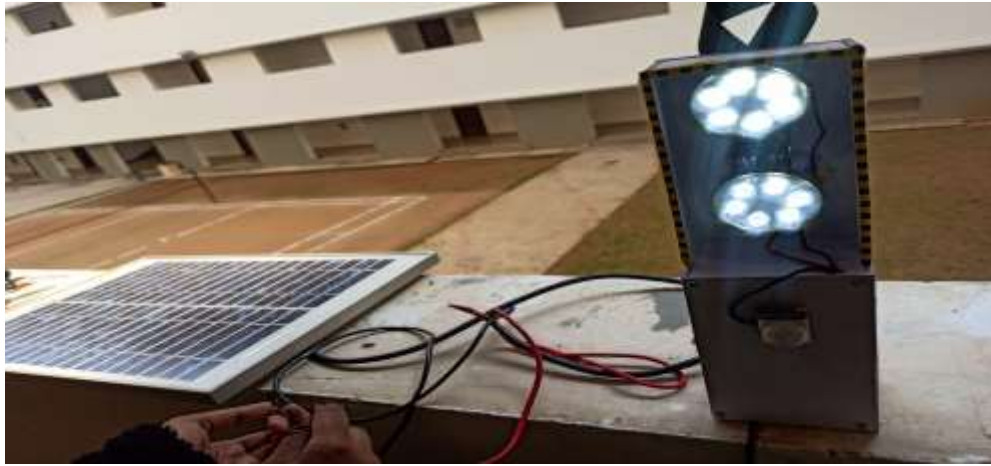
Fig. 2. Dynamic solar PV lighting system
